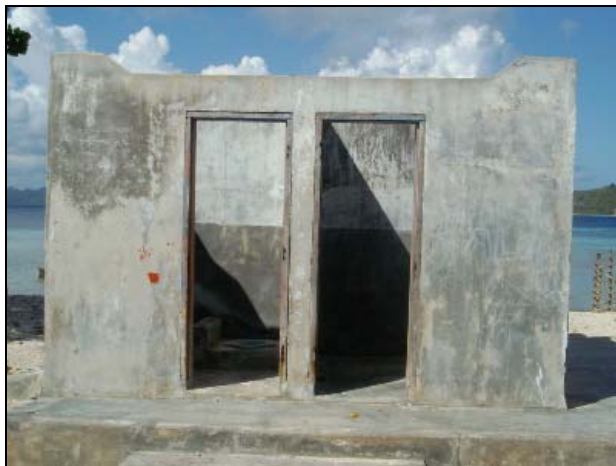
MCK with no water supply, never used
