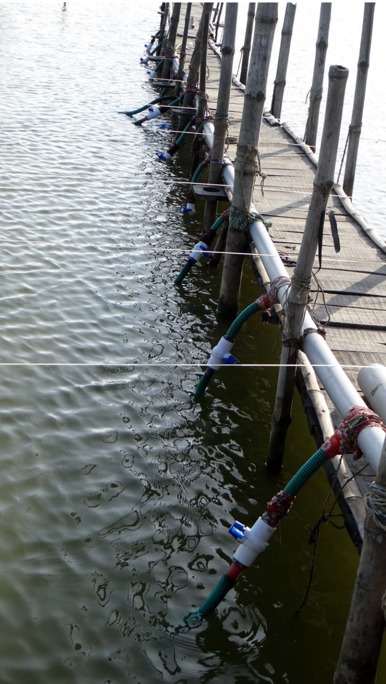
Several units are interconnected using the main pipe from the pump.
