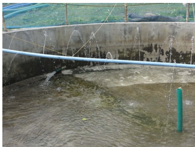
PVC pipes as aeration device, used by Sri L. Barman.
