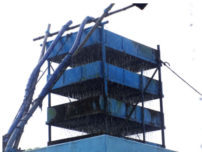
Cascade aerator above overhead tank.
