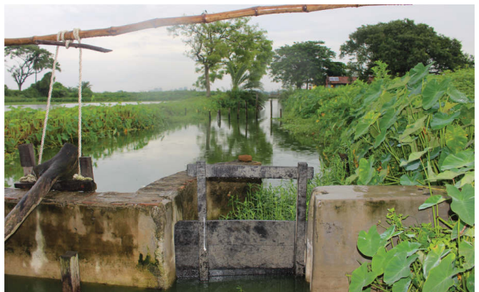
Indigenous switch-gate in the sewage feeder channel to regulate inflow to fish ponds.
