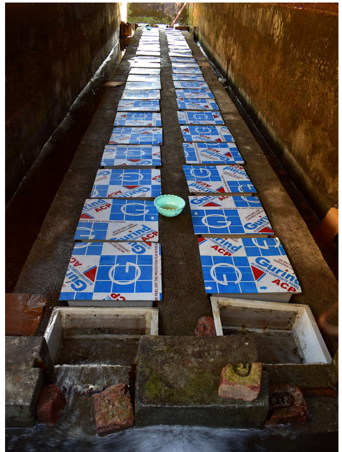
Concrete channels for trout seed rearing at Bairangana.
