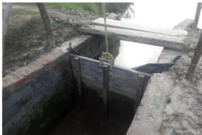
Sluice gate or water gate with wooden shutter in a bheri.
