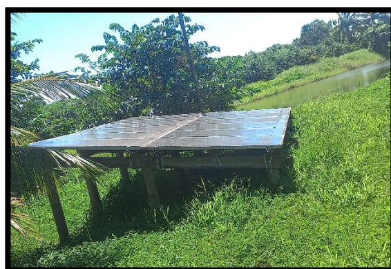
Figure 2. Current solar panel system at SEAPAC farm.
