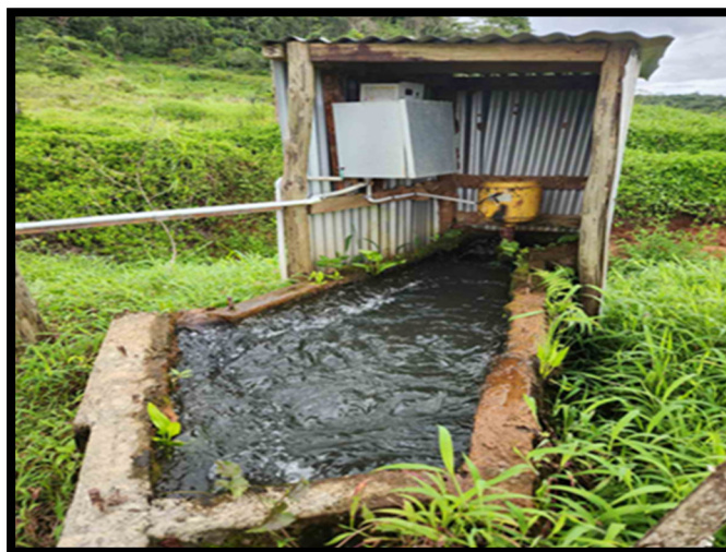
Figure 3. The current 3kw hydro turbine system at Growa Fish Farm, whilst the farm is in the process to upgrade this to a 5Kw.
