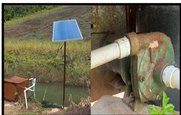
Figure 1. Solar water pump in operation at Growa Fish Farm
