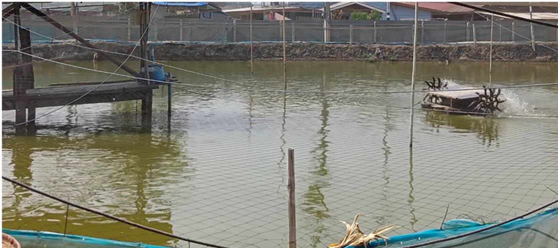
Figure 2. A Four-blade solar power aerator turbine (350 Wp) installed in each fish rearing pond.
