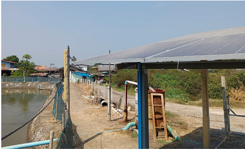
Figure 1. Solar power system (solar panel 8.05 kWp) for water pumping.
