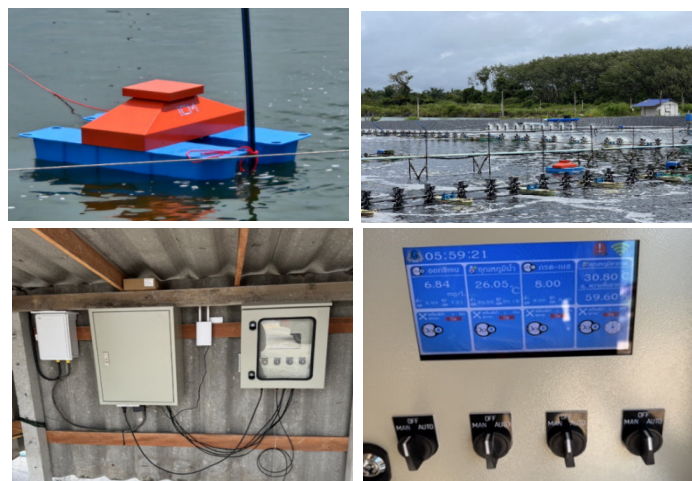
Figure 3. Smart aerator control installed in a super intensive white shrimp farm with a real-time display screen.
