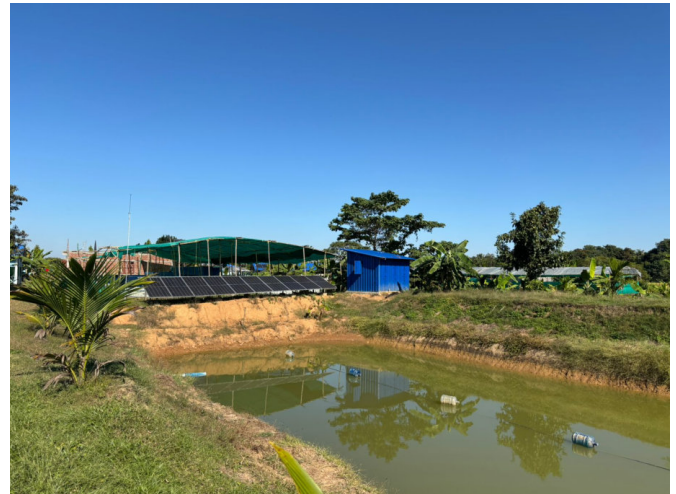
Solar panel for electricity supply.
