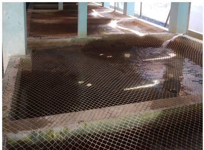
Ante tank / storage tank.
