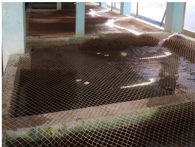
Ante tank / storage tank.
