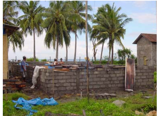
Concrete blocks being used to construct rearing tanks for a small hatchery in Bali, Indonesia.
