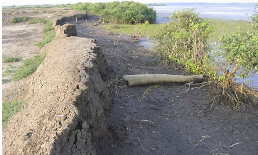
Flood damage to ponds in Dhabharevu. Ponds without the protection of a mangrove buffer suffered severe damage. Areas protected by mangrove fared much better (note the lesser damage to the dyke in the background).
