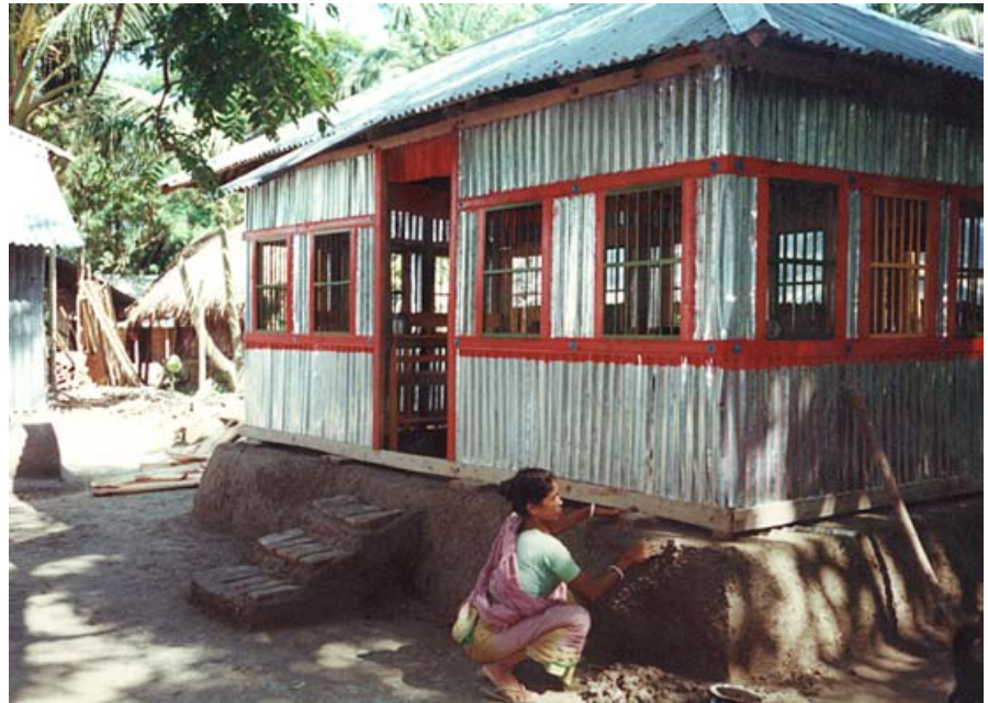
A tin shed based house is an indicator of the wealth status of family. A Gher farmer is finishing the house built with income earned from Gher farming
