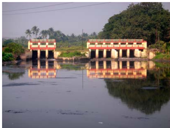
The regulator gates at Bantala which control the level of wastewater in the main canal.
