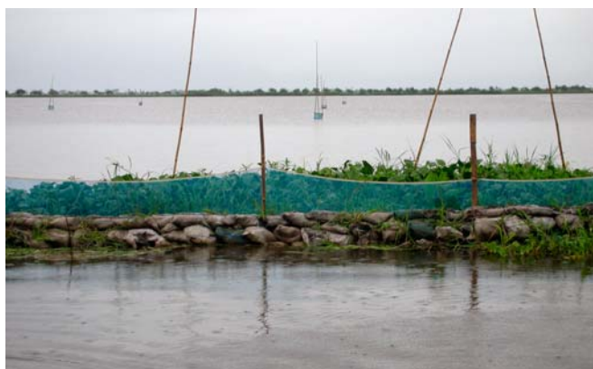
A fish pond dyke breached by Nargis repaired with earth filled sacs.
