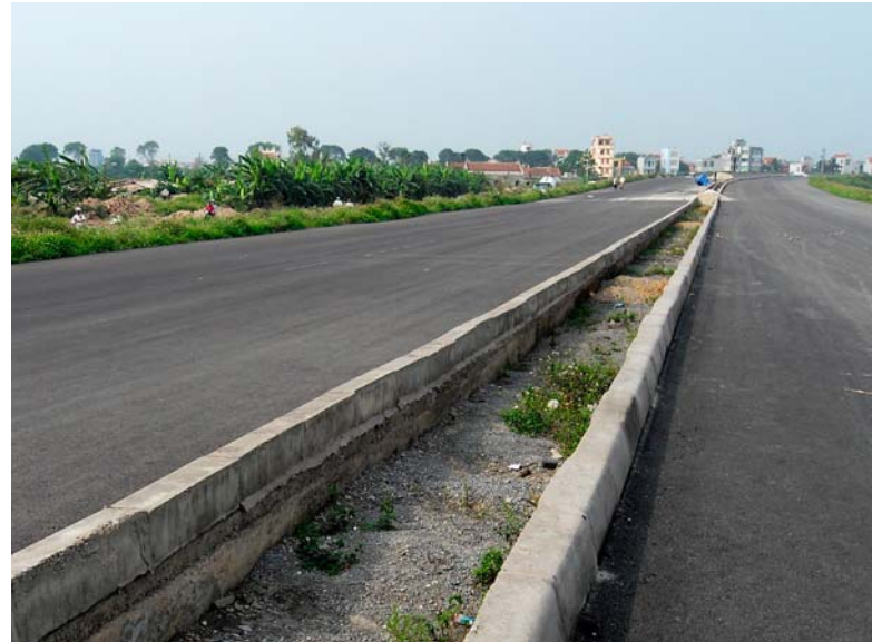
Major highways are being constructed through the wastewater-fed aquaculture area in Thanh Tri District, Hanoi.
