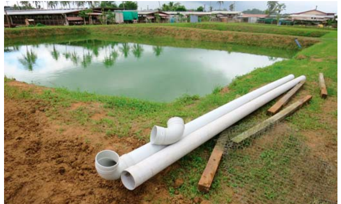
Swivel stand pipes used for pond drainage.
