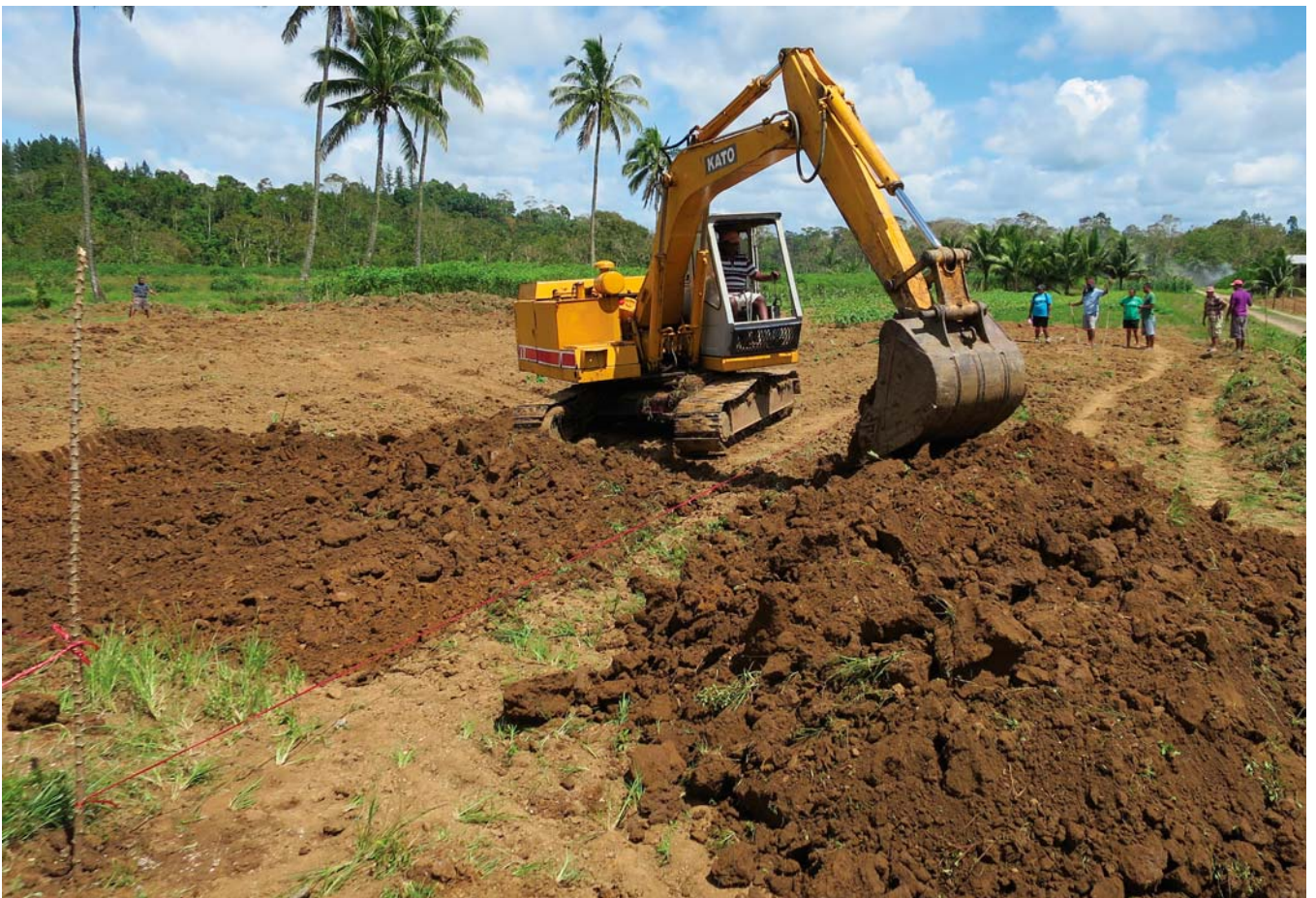
Starting to dig down into the pond bottom area to remove soil to build a dike.
