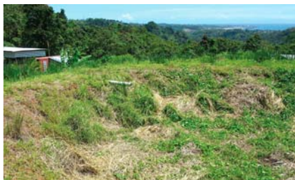
Hillside pond that did not hold water, Homes of Hope.
