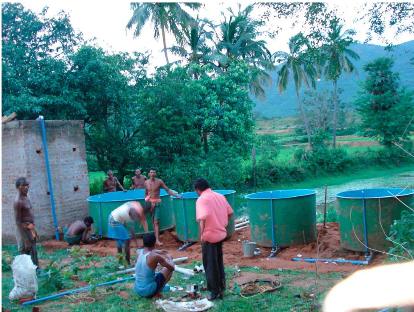
Fiberglass reinforced plastic carp hatchery installation in Khanguri Village.
