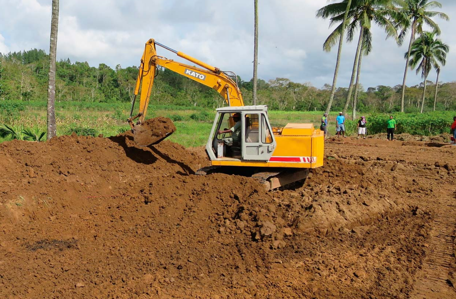
Continued removal of soil from the pond bottom area to form a dike.
