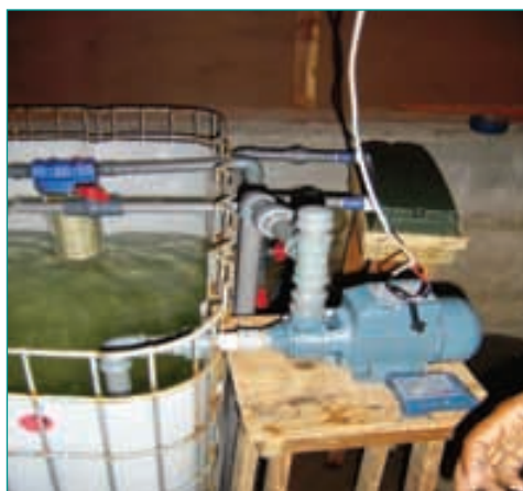
High-tech water recirculation system
