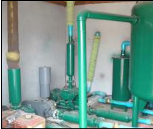
Figure 7: Air blower at KCFRDC
