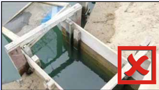
Improperly fixed water filter net
