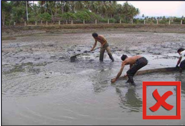
Improper removal of black soil
