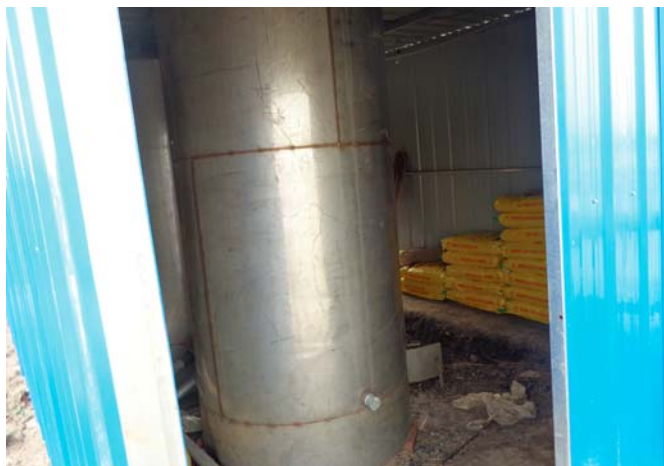
The boiler used to heated water.
