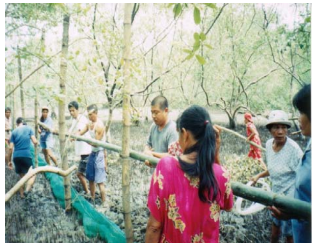
NMPC women taking an active part in the construction of a mudcrab pen during the three-day training
